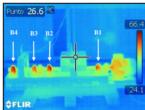
Fig. 3. Thermography image of the platform after 45 minutes: two inertias, motor 1 directly connected to the grid.
