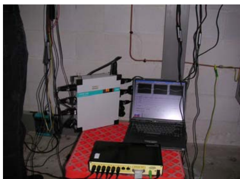
Fig. 5. Inasus Factory with the different instruments for make the comparison of the results of power quality measure.
