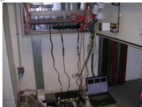
Photo 1. Unilyzer 812 installed at the control panel.
